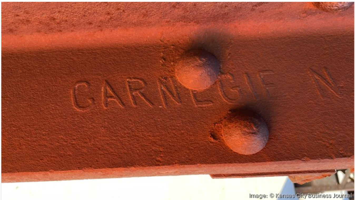
The Rock Island Railroad Bridge was constructed in 1905 using steel from Carnegie Steel Co.
